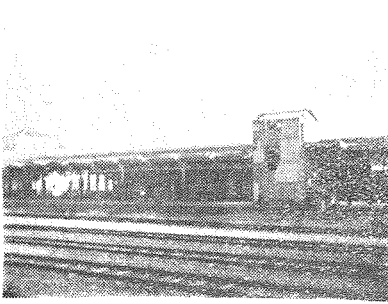
高雄站第一月臺電梯房屋頂牆壁颶風吹破 Destroyed elevator room of railway platform at Kaohsiung.
